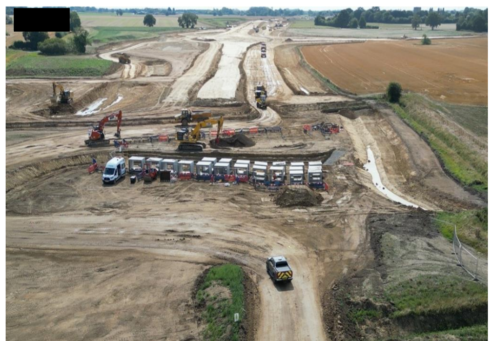
Facing South – Drainage culvert installation (foreground) and Bypass carriageway approaching Parkers Lane roundabout (background, center)
